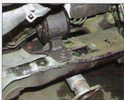
This HCP Engineering rear engine mount has been bolted into place after the rear crossmember lip was pounded down flat. It's better to flatten it too much than not enough so that the bracket won't fit.
